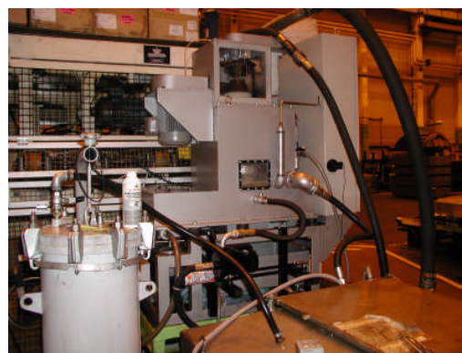
Centrifuge installed in Line 51
